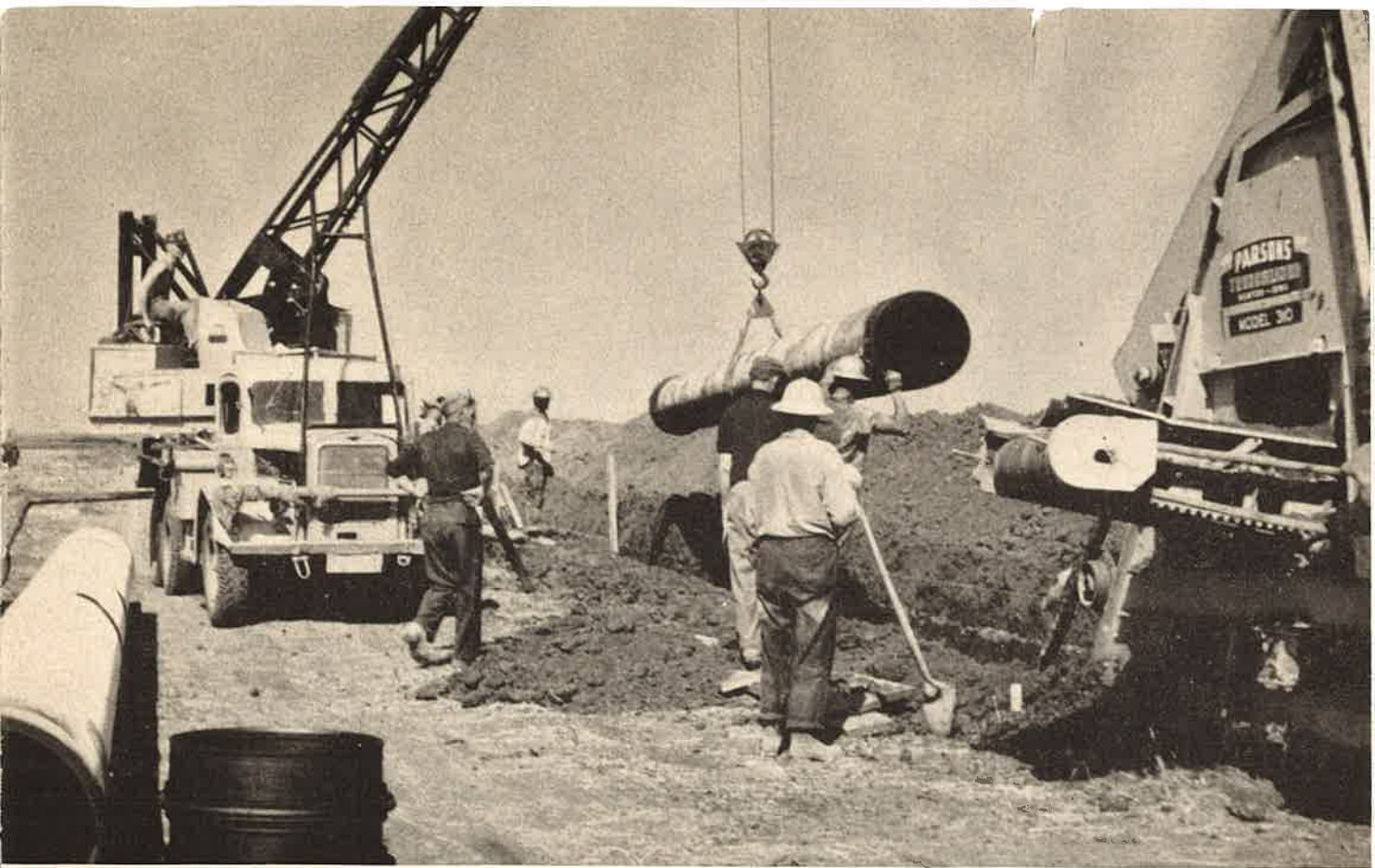
LAYING OPERATIONS on the Armco 24-inch Welded Steel Water Line followed directly behind the trencher. Better than 12 miles of pipe was used from the filtration plant to Moose Jaw.—PHOTOS BY R. O. HAYES
